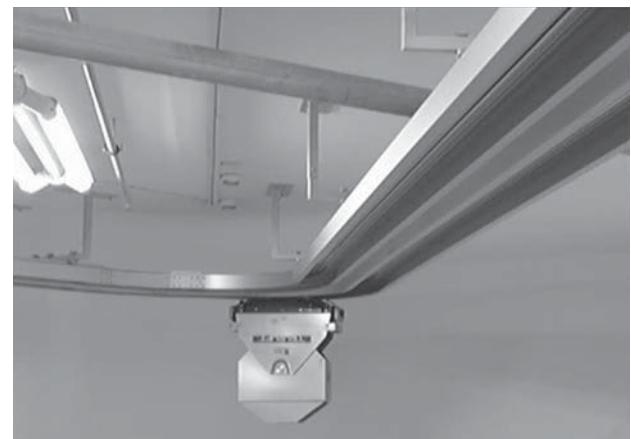
Figure 6. The Telelift system.
